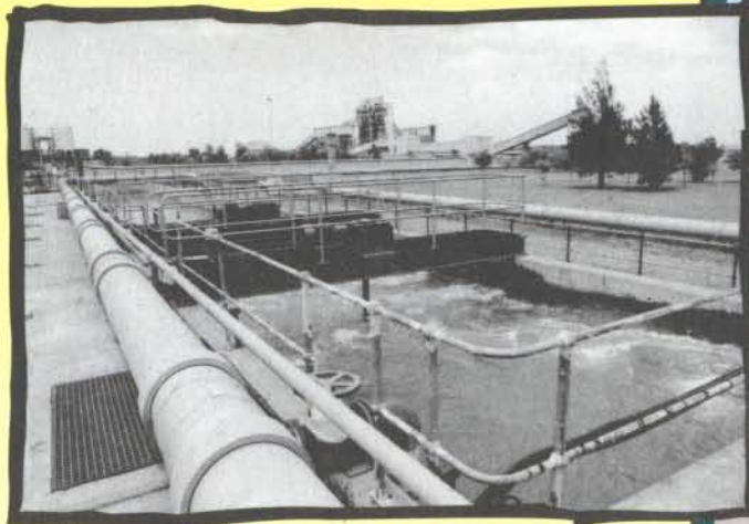
A CARBONATION TANK
